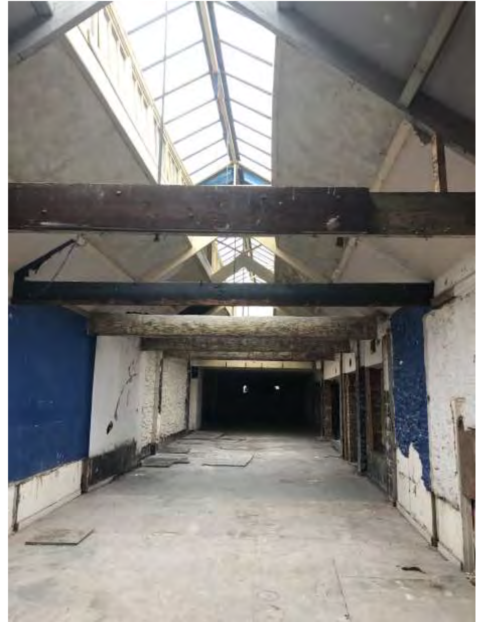
Existing vacant, dilapidated space behind the High Street
