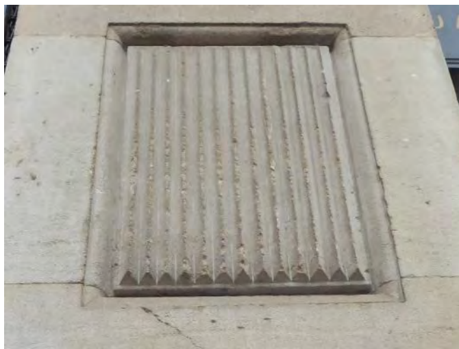
Figure 12 Panelled detail to pilasters on ground floor of arcade entrance block on High St.
